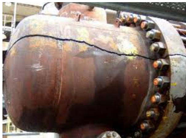
Figure 1: Nozzle side failure of a shell and tube heat exchanger.
