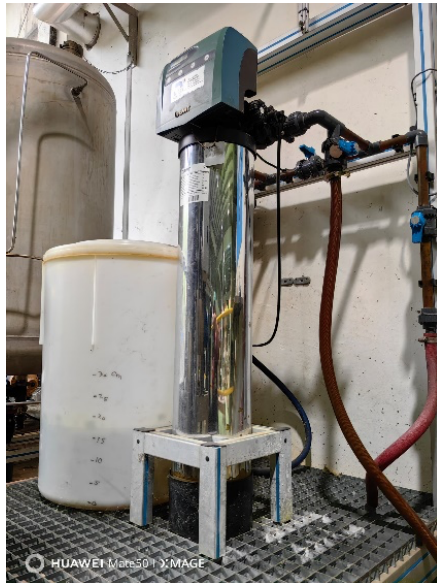
Figure 2: External Water Treatment Unit at Water-Tube Steam Boiler (water softener)
