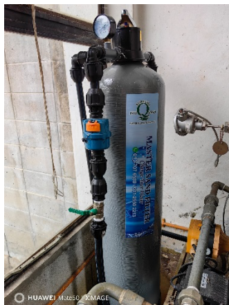
Figure 1: External Water Treatment Unit at Water-Tube Steam Boiler (sand filter)
